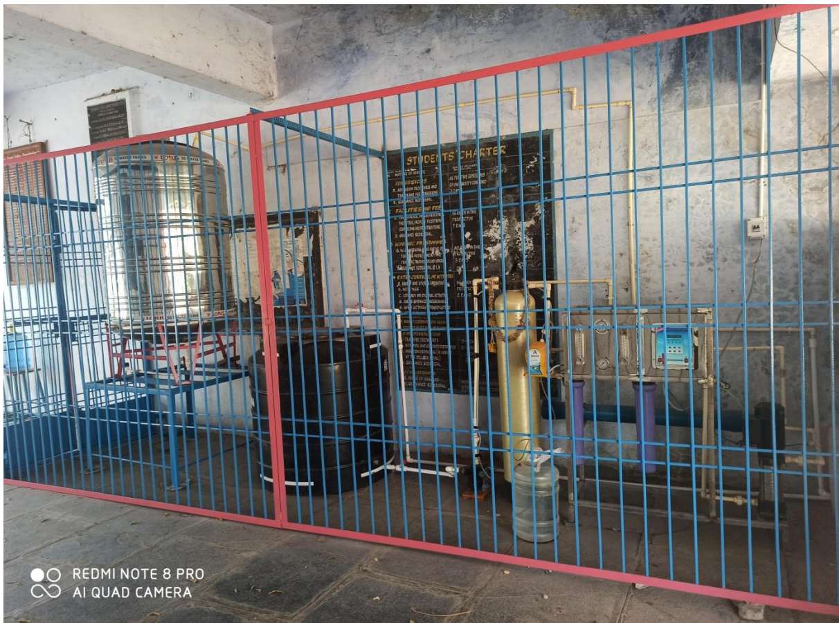
A new RO water plant installed in the college
